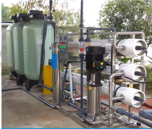
RO Pure Water Cap. 10Ton/Hr (Quanzhou-Fujian)
